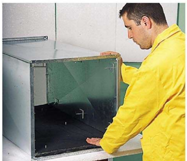
Apply the shaped Duct Liner over the mechanical fastener pins. Fit the washers or caps to pins and snip off excess shank of pins.
